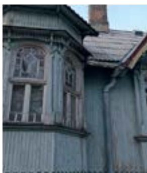
High and low-resolution photograph of a facade element (author: J. Heinsbergs)
